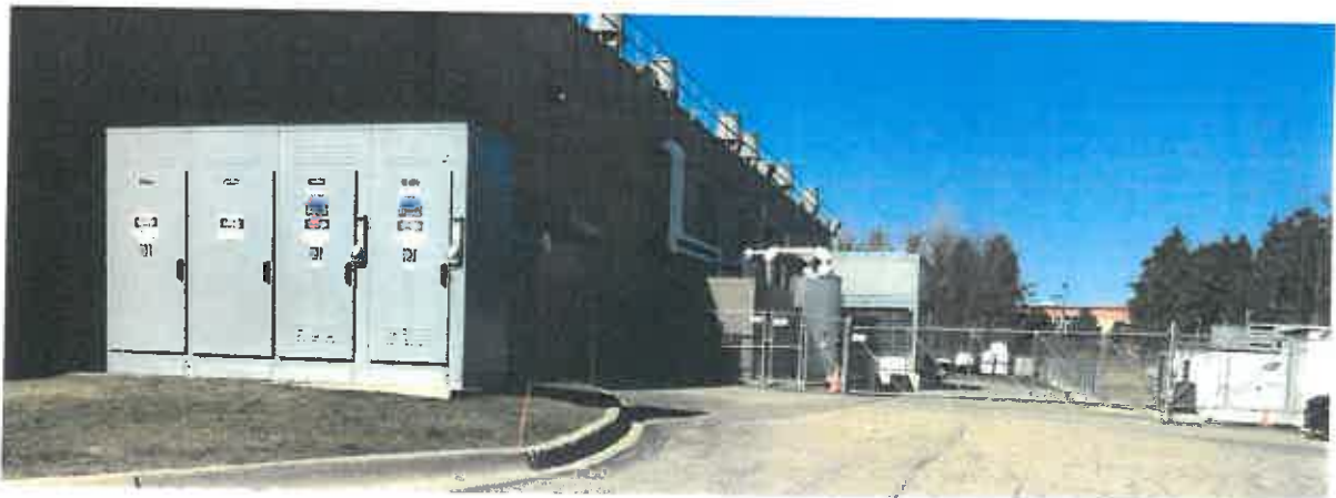
EQUIPMENT IMMEDIATELY ADJACENT TO WEST PROPERTY LINE OF BECK ROAD RESIDENCE HOTEL SITE
